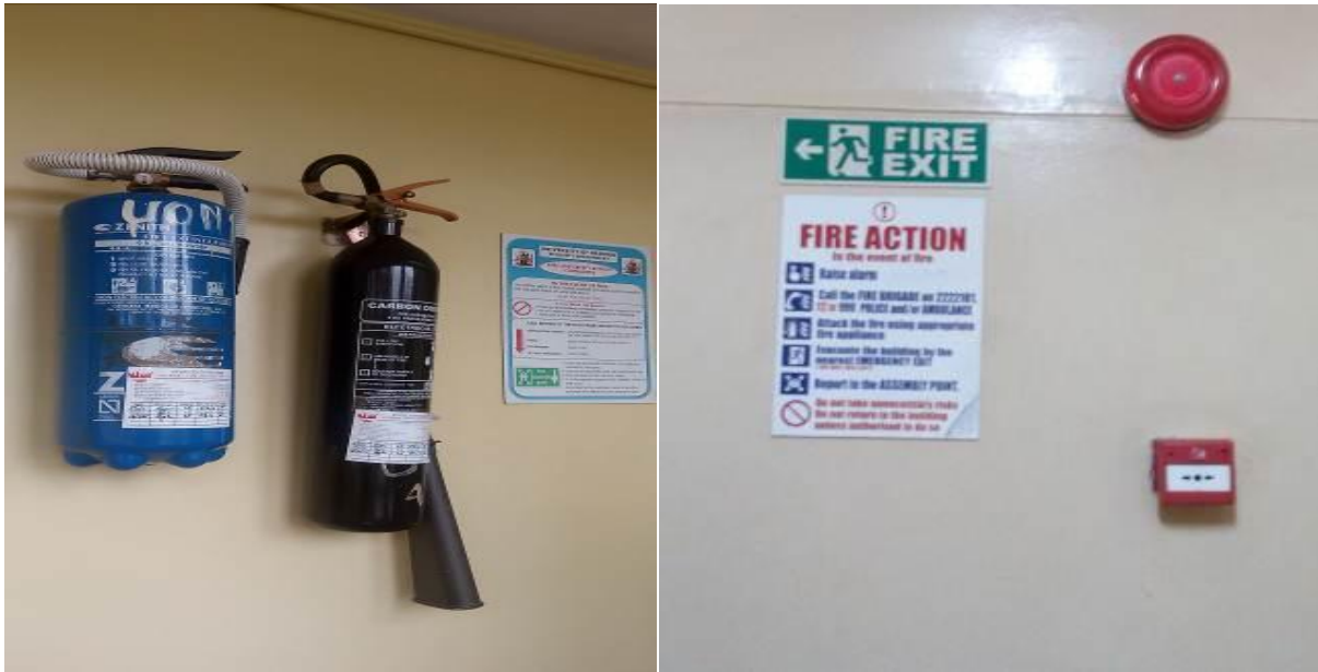
Plates 1 and 2: Fire extinguishers and a ction card strategically placed
