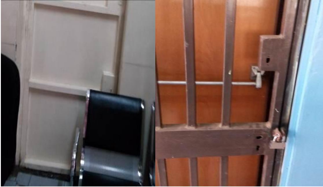
Plates 7 and 8: Locked and obstructed exits
