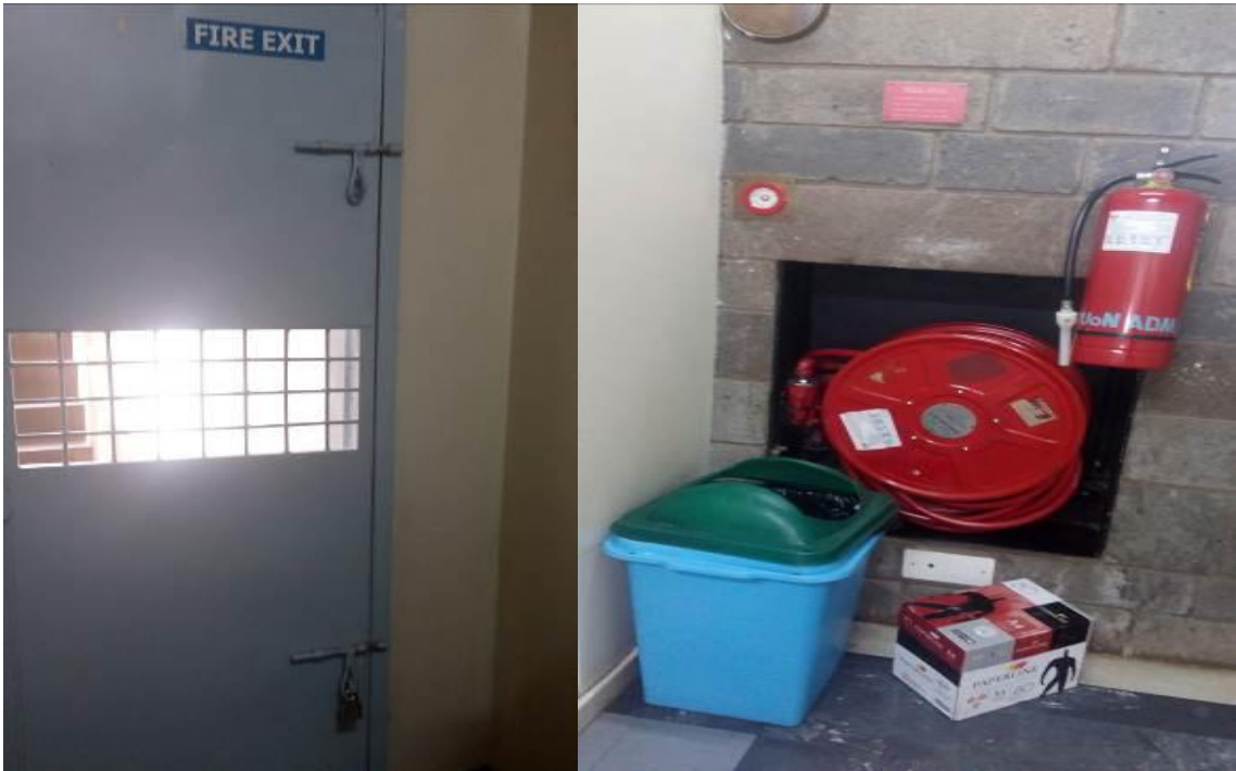
Plates 9 and 10: Locked fire exit and obstructed hose reel.
