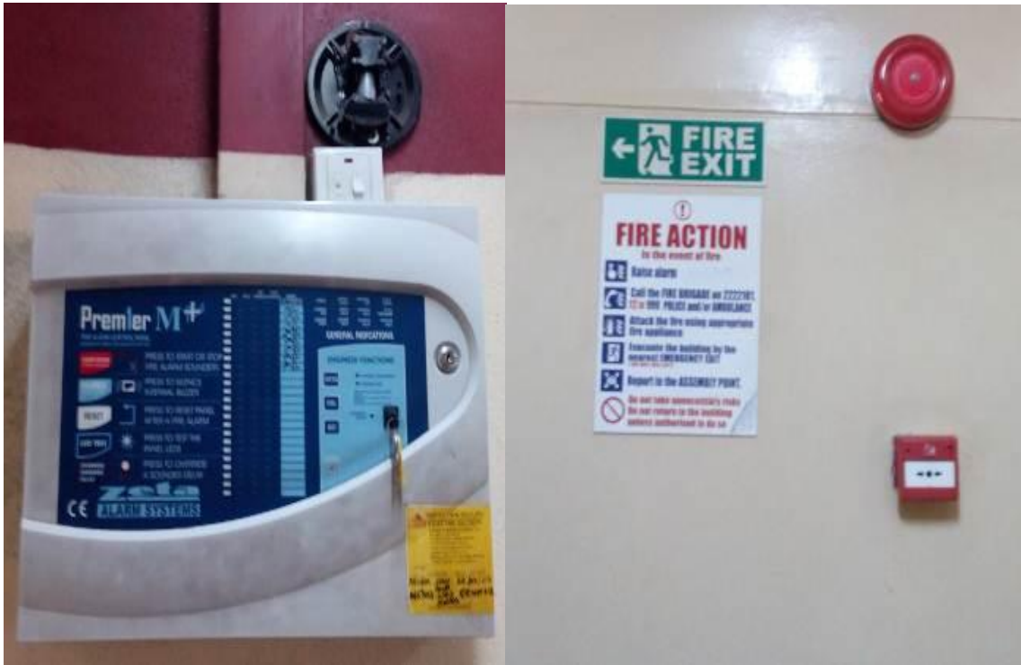
Plate 11 and 12: A Non-functioning Fire Alarm Control Panel with a call point, exit signage and fire action card
